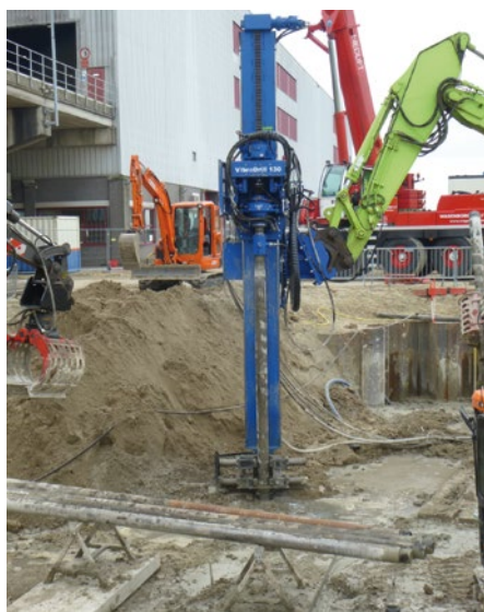
VD100 drilling in sand and gravel, 65 m deep, hole diameter 190 mm, flushing with water
